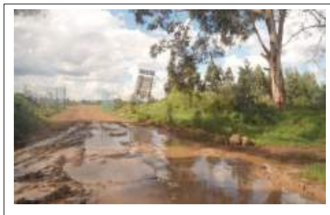
Plate 6-12: Poor state of the access road to the dumpsite
