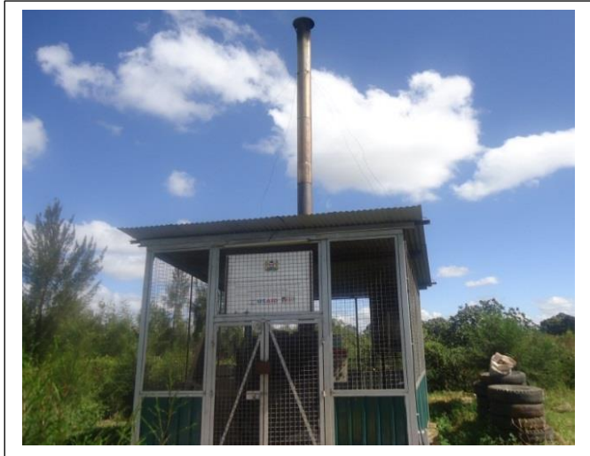
Plate 6-14: Nanyuki District Hospital Incinerator
