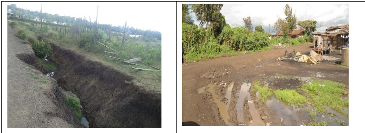
Plate 6-5: Lack of storm water drains in Muthaiga and Majengo areas
